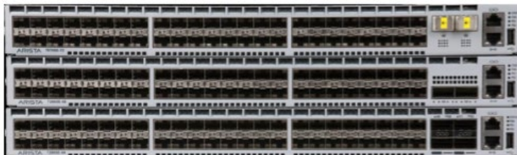
Figure 6: Arista 7280E Series Switches
